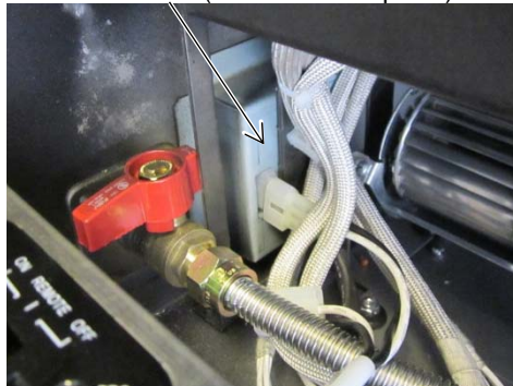
Junction Box (from inside fireplace)
