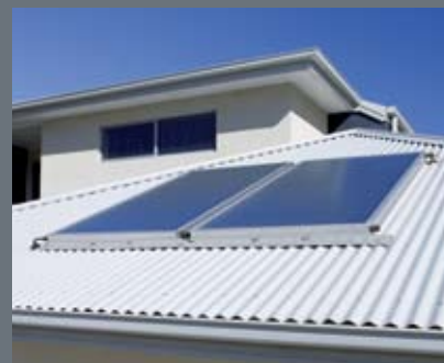
Gas Boosted Solar Hot Water
